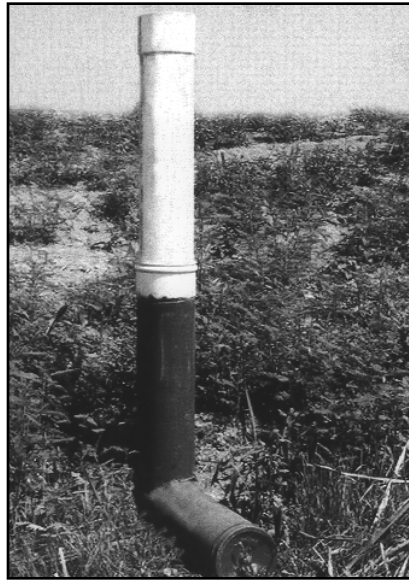
Figure 3. Outside drain fitted with a "T-stand pipe" and alfalfa valve.
